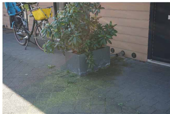
Figure 7 | Case #8 has been assigned the root cause actual use of SUDS. A flowerpot was placed in front of a dwelling's water outlet, preventing water to be discharged properly.
