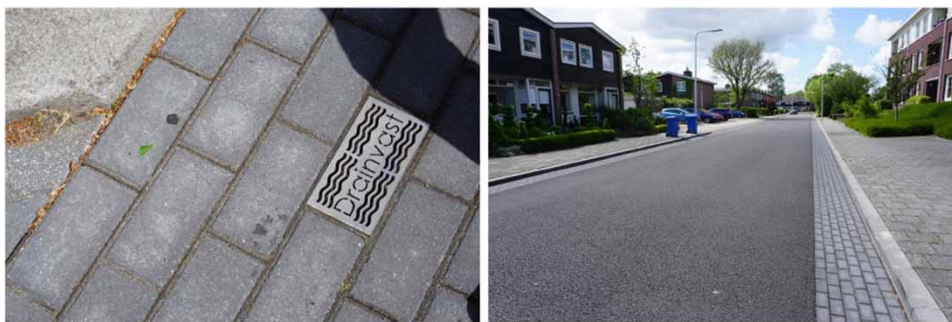
Figure 6 | Case #33 has been assigned the root cause Incomplete knowledge about the internal technical processes. The pavers were separated by joints filled with a permeable material, allowing water to infiltrate. Even after a small rainfall event, however, water remained ponding for at least 1 h. As such, it was thought that the permeable material had become clogged, leading to a malfunction of the SUDS.
