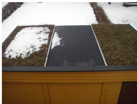
Figure 2 | Uneven snow melting from the three experimental roof plots (GR1 to the left). Photo: April 2, 2010.
