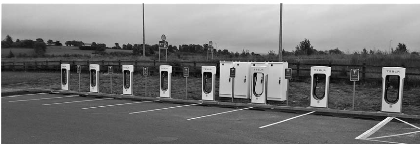
Figure 4 Eight-bay Tesla super charge site in Birdhill, Ireland, requiring 4 \times 135 kVA grid connections, i.e. in excess of 0.5 MVA of grid connection. Photographer: Thomas Conway.
