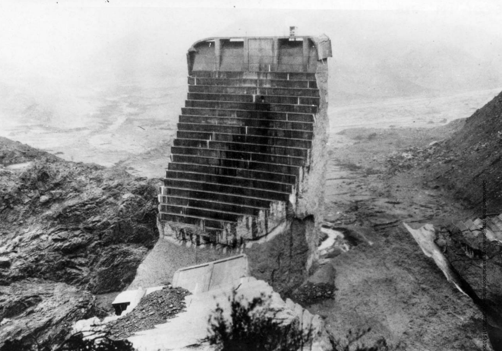
The remains of St. Francis Dam. COURTESY OF THE LOS ANGELES PUBLIC LIBRARY PHOTO COLLECTION.
