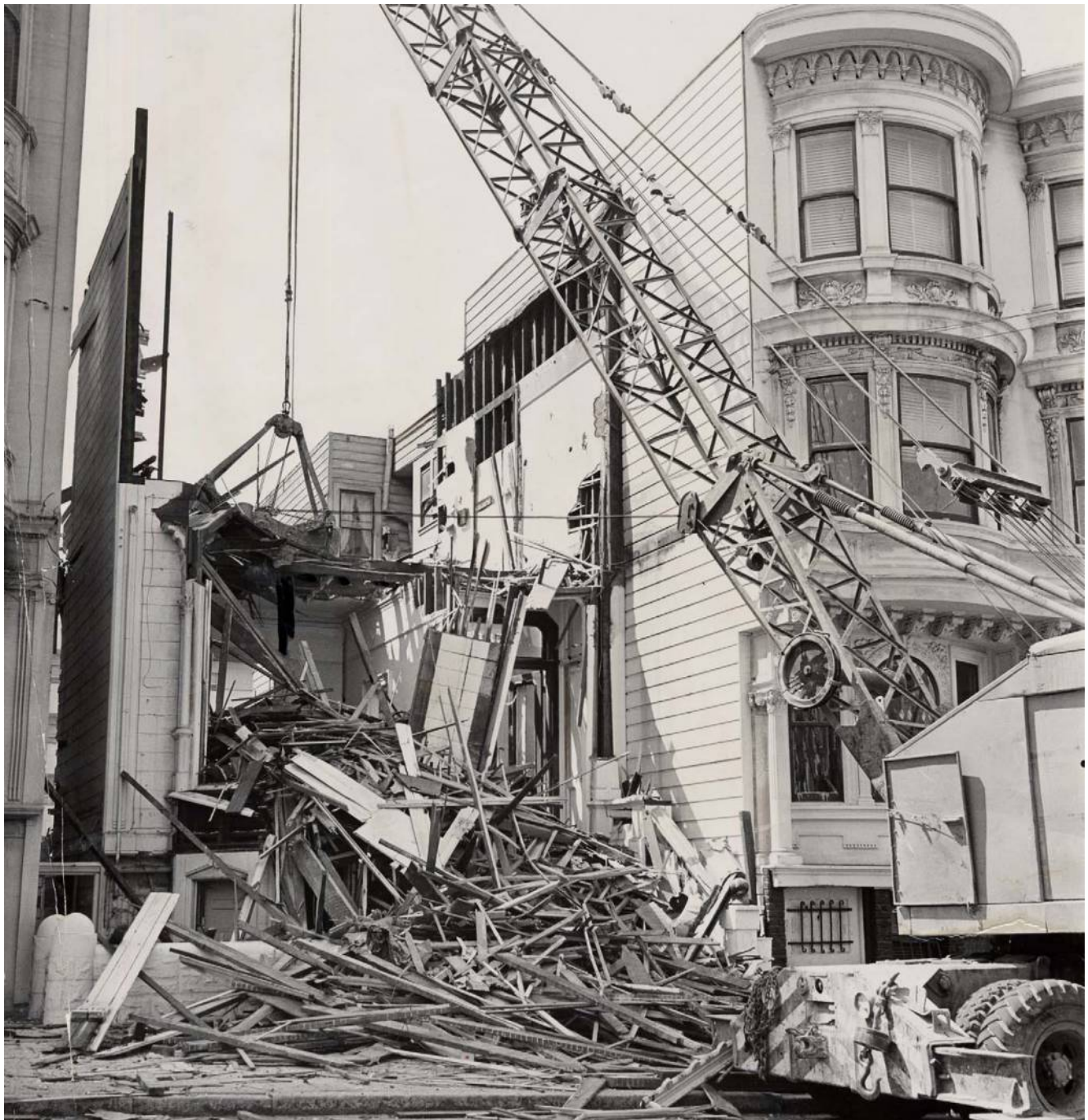
This photograph ran in the San Francisco Examiner with the caption “A huge crane smashes into kindling wood one of the blighted dwellings in the 1300 block of Ellis St. as the city steps up its war against slums in the Western Addition.” COURTESY OF SAN FRANCISCO HISTORY CENTER, SAN FRANCISCO PUBLIC LIBRARY.
