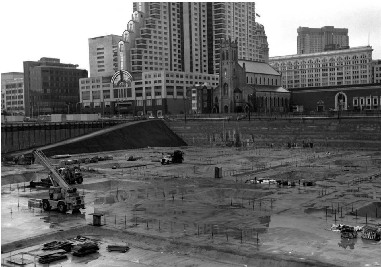
Construction site of the Yerba Buena Center and convention hall, Marriott Hotel in background, South of Market district. COURTESY OF DAVE GLASS.
