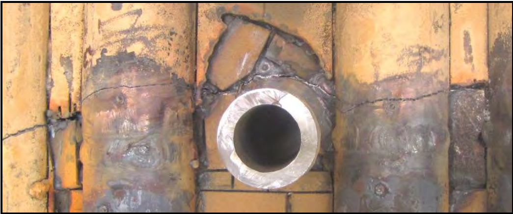
Figure 9: Brittle Fracture through T23 Swages and T23 Welds in the Vicinity of High Crown Seals
