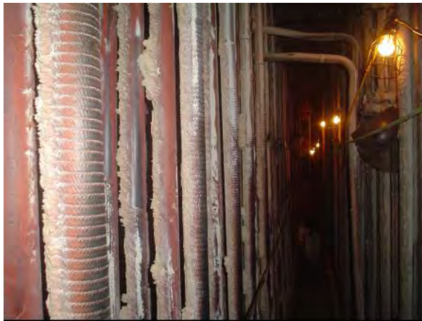
Figure 5. SA213-T2 super-heater tubes overlaid with filler metal 72, after 7 years of service in AEP's Rockport #1 plant.
