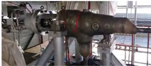
Fig. 22 Turbine control valve (before thermal insulation) (Courtesy of Fuji Electric)
