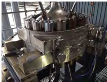
Fig. 23 Turbine casing without thermal insulation (Courtesy of Toshiba)
