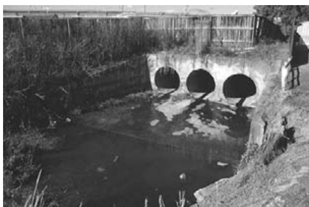
Photo 3. Domestic cats were recorded repeatedly preying on bats roosting within this stormwater drain at Blacktown. No bats have been recorded using this roost during recent years.
