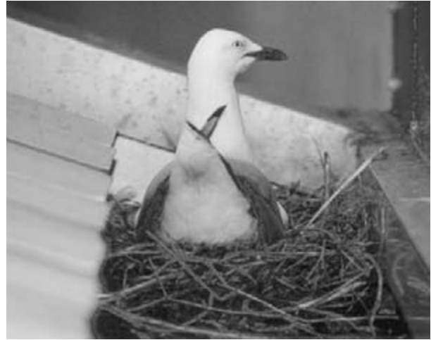
Figure 3. Typical Silver Gull nest site on roof, blocking gutter
