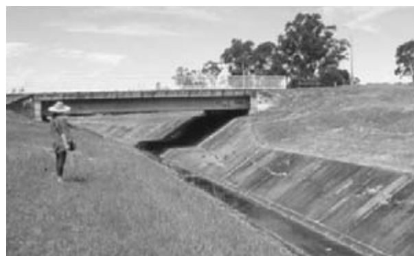
Before restoration - Clear Paddock creek in 1995 - a bleak concrete-lined storm water channel. Photo: M. Crawford
