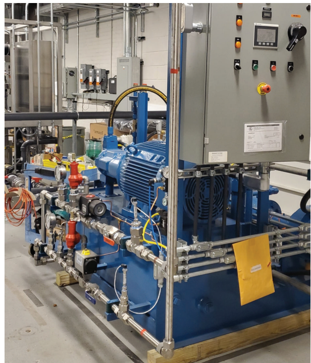
Fig. 14 Pilot-scale HPSG using low-speed reciprocating compressor
