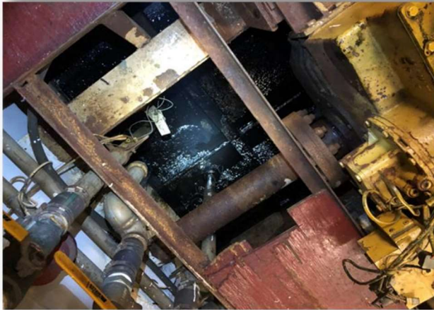
Figure 5: Machinery Space Bilge with oily waste
