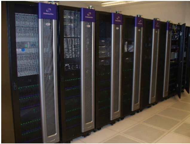
Figure 5. U.S. Library of Congress National Audio Visual Conservation Center: Data Center.
