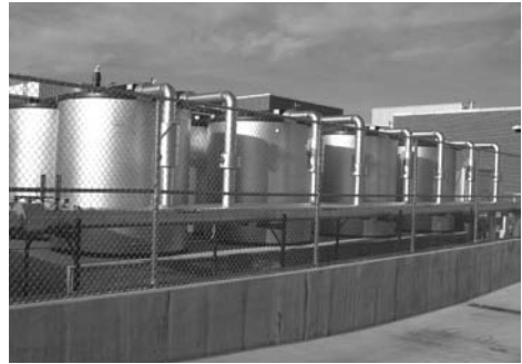
Ice storage tanks.
