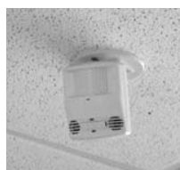
FIGURE 5. Watt Stopper DT-200 energy-saving motion and light sensors are installed in the classrooms.
