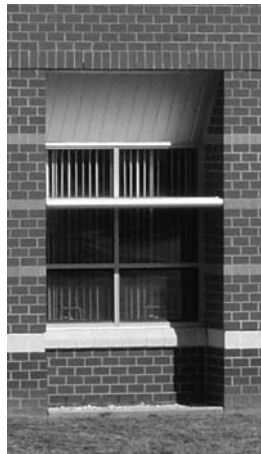
FIGURE 3. Light shelves and angled soffits maximize and redirect daylight upward through the windows to light-colored ceilings.
