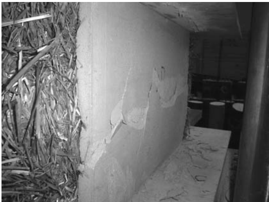
FIGURE 12. Typical failure of on-edge, plastered straw bale.
