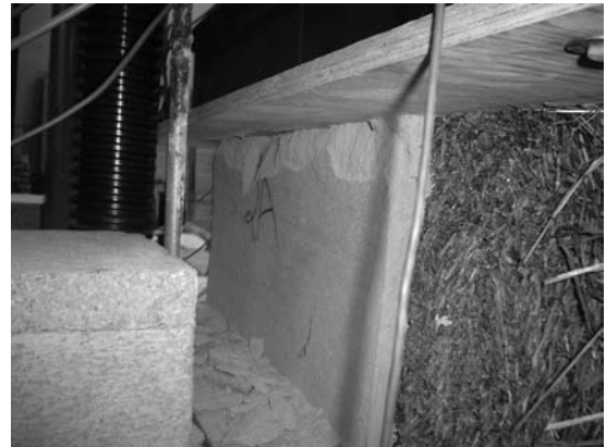
FIGURE 10. Typical failure of a flat, plastered straw bale.
