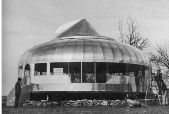
FIGURE 1. The Dymaxion (Wichita) House at the construction site, upon finishing the outer shell. (Source [5])
