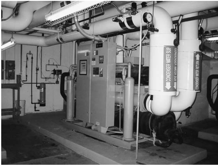
FIGURE 6. One of the two 125-ton chillers at the Columbus Museum of Art. Each has the capacity of a 200-ton chiller when used in tandem with the stored ice. (Photo courtesy of Schooley Caldwell Associates.)
