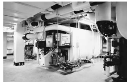
FIGURE 4. In the Ohio Statehouse, chiller-heaters offer space savings because they use less floor space; in addition, they had the advantage of being able to fit into a very tight head space of just over 100 inches. (Photo courtesy of Schooley Caldwell Associates.)
