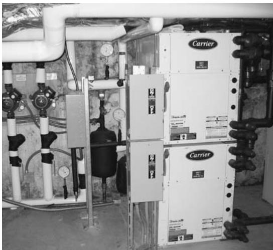
FIGURE 10. The indoor heat pump unit at the Westcott House with three zone pumps.
