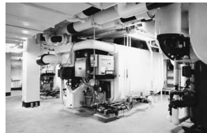
FIGURE 4. In the Ohio Statehouse, chiller-heaters offer space savings because they use less floor space; in addition, they had the advantage of being able to fit into a very tight head space of just over 100 inches. (Photo courtesy of Schooley Caldwell Associates.)
