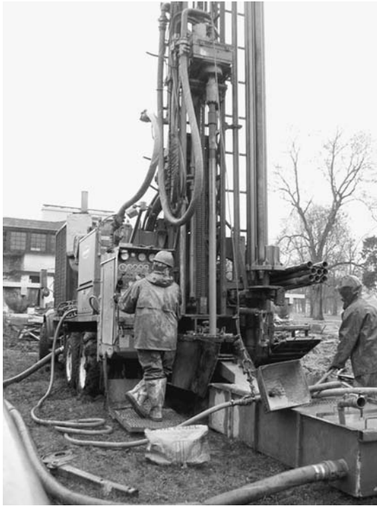
FIGURE 9. At Westcott House, the design used 22 vertical deep wells—14 in the front yard serve the main residence, and 8 in the back yard serve the carriage house. (Photo courtesy of Schooley Caldwell Associates.)
