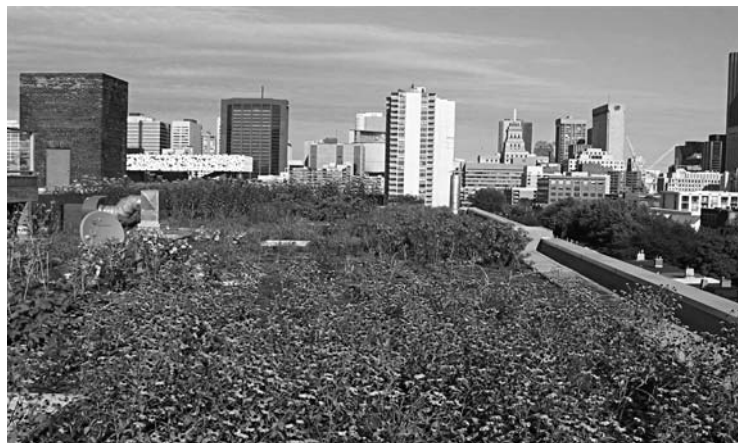
FIGURE 2. Extensive green roof on top of the J.A. Robertson Building, 215 Spadina, Toronto, Ontario. This is one of two buildings owned and operated by Urban Space with green roofs. The green roof features a mix of flowers and grasses. The photograph was taken from the fifth floor observation deck, facing east. Figure is provided courtesy of Beth Anne Currie, Centre for Social Innovation, Toronto, ON.
