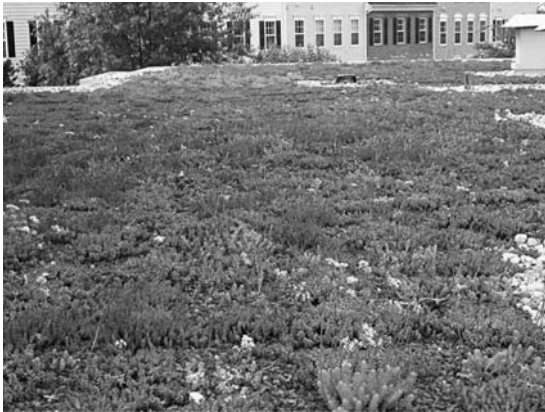
FIGURE 3. An extensive green roof planted with sedums is located on Yorktown Squares Condominiums in Falls Church, VA. This EnviroTech Greenroof System from Building Logics, was the award winner in the Extensive Residential category at the 4th Annual Greening Rooftops for Sustainable Cities Conference and Trade Show in Boston, MA. Courtesy of Green Roofs for Healthy Cities. www.greenroofs.org .
