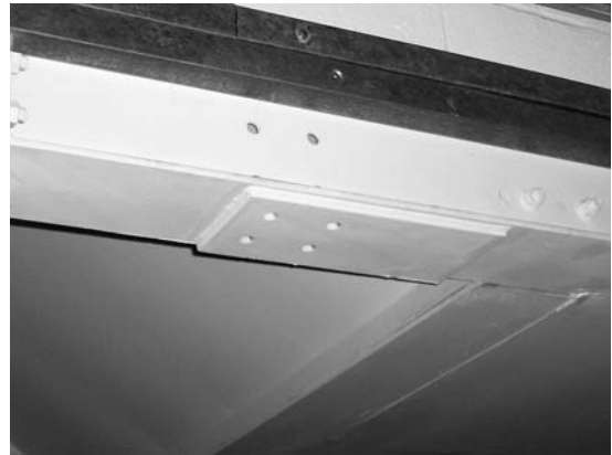
FIGURE 3. Steel with plates left from its previous use.
