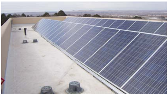
48 panel 10 kW photovoltaic system.
