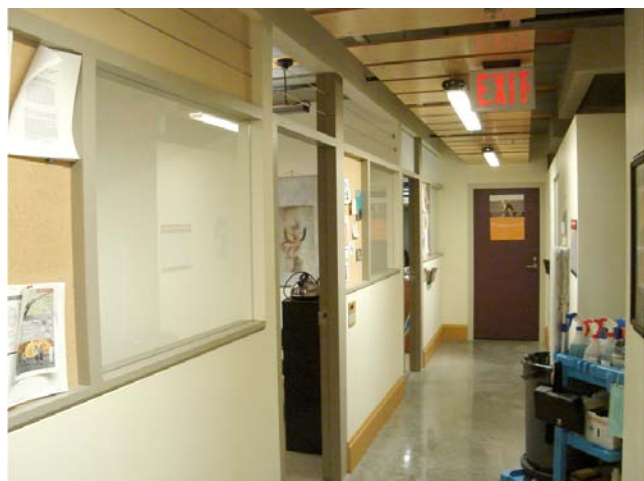
FIGURE 2. Large openings above doorways and corridor partitions.
