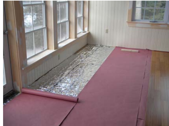
Radiant barrier under 3-season room floor.
