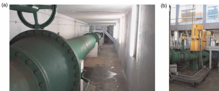
Figure 2 | Novara pumping station: (a) the pipe inside the station; (b) the pumps.
