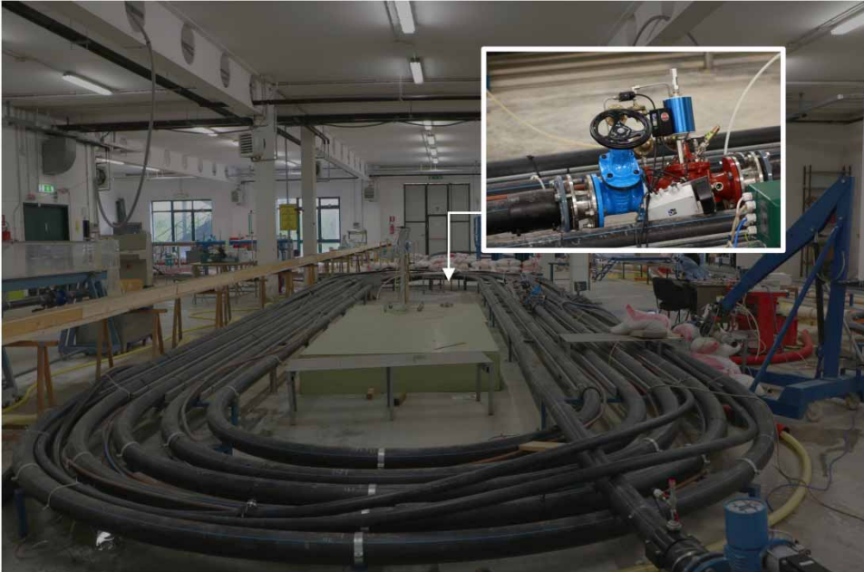
Figure 2 | The experimental pipe and the PRV (in the insert) at the Water Engineering Laboratory (WEL) of the University of Perugia, Italy.
