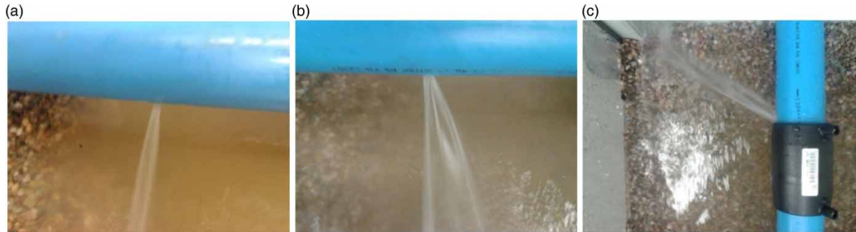
Figure 3 | Photographs of leaks: (a) round hole; (b) longitudinal slit; (c) electrofusion joint.
