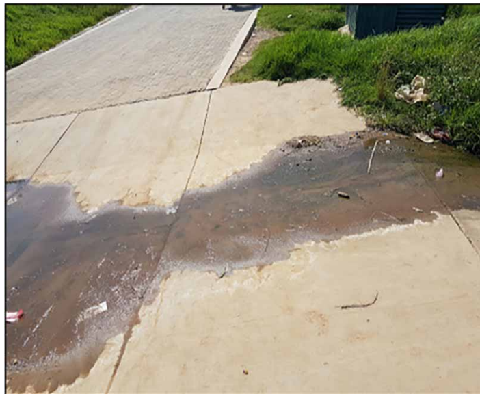
Figure 4 | Water from broken pipe flowing in the street in QwaQwa (Source: Authors).
