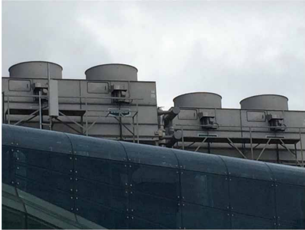
Figure 1 | Open recirculating CTs.
