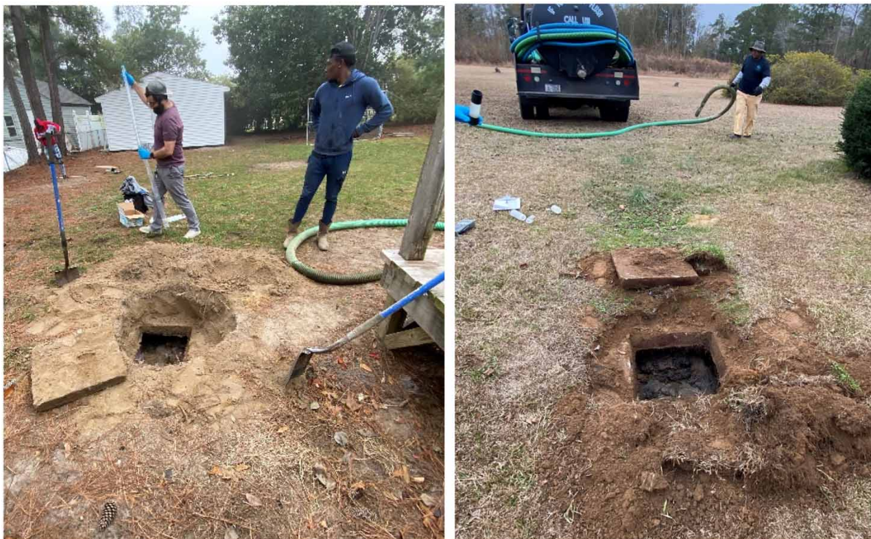
Figure 2 | Septic tanks were uncovered to allow for collection of wastewater samples (left image) and to pump the septage from the tanks using a pump truck and suction hose (right image).
