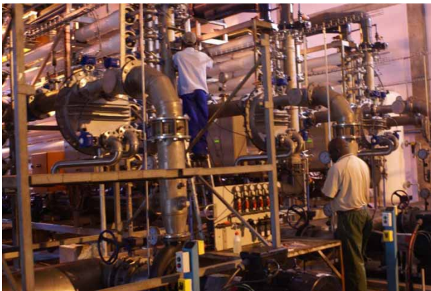
Figure 2 | NGWRP – Ultra-filtration undergoing servicing by local staff.
