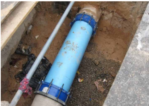
Figure 5 | Lined pipe sections connected by PVC pipe (with permission from Matthews et al. 2015).
