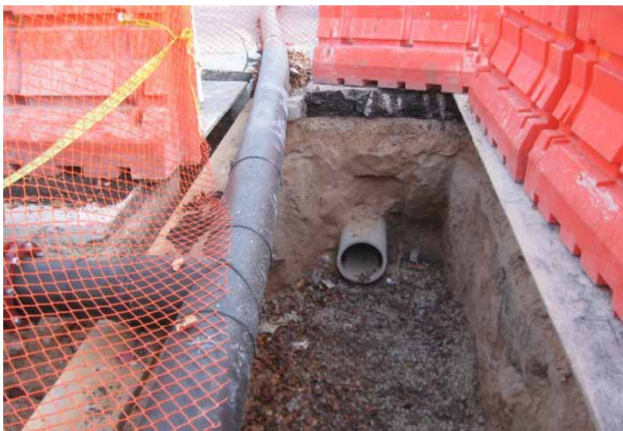
Figure 2 | Access pit with pipe removed (right) and bypass (left) (with permission from Matthews et al. 2015).
