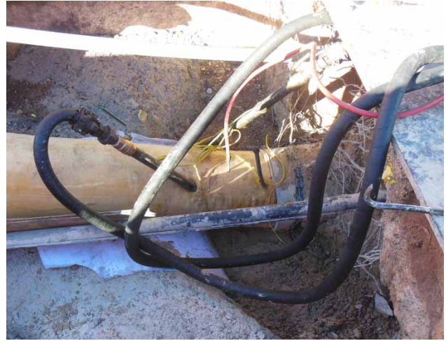
Figure 3 | Liner punctured by stingers at Station B.
