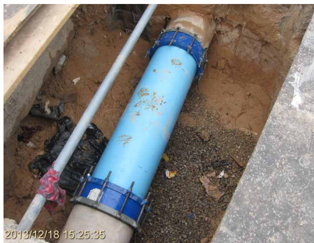
Figure 5 | Lined AC pipe sections connected by PVC pipe.
