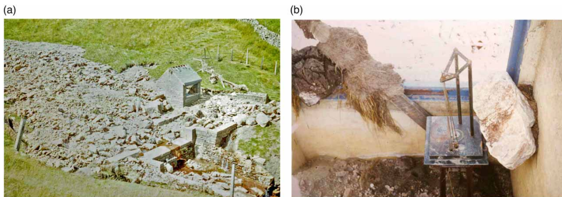
Figure 2 | (a) The gauging structure on the West Grain showing the boulder accumulation, the damaged gauging hut, the swash mark on the grass and the normal summer low flow. (b) The interior of the gauging hut from the destroyed roof with the level recorder pinned down by a boulder.
