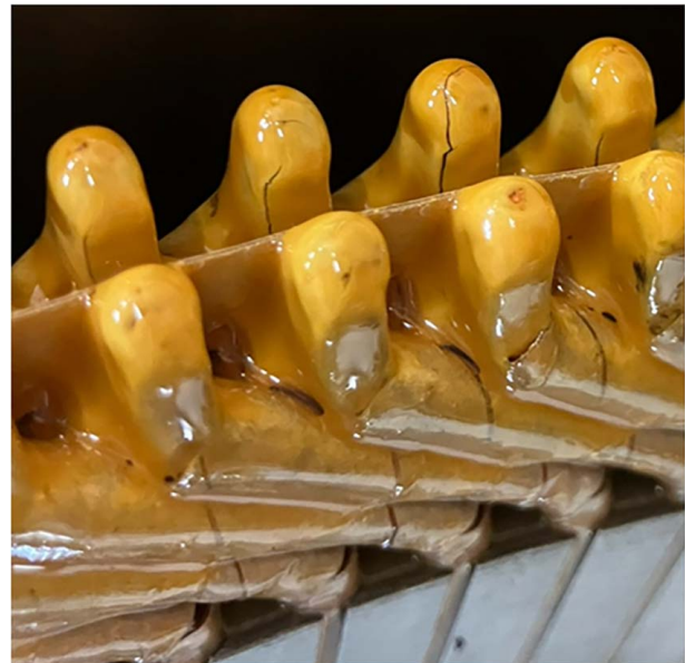
Fig. 7 Cracks in the insulation layers in unit 5
