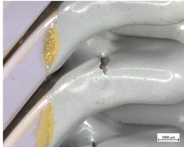
Fig. 6 Crack on the polymer coating close to the weld area in unit 2
