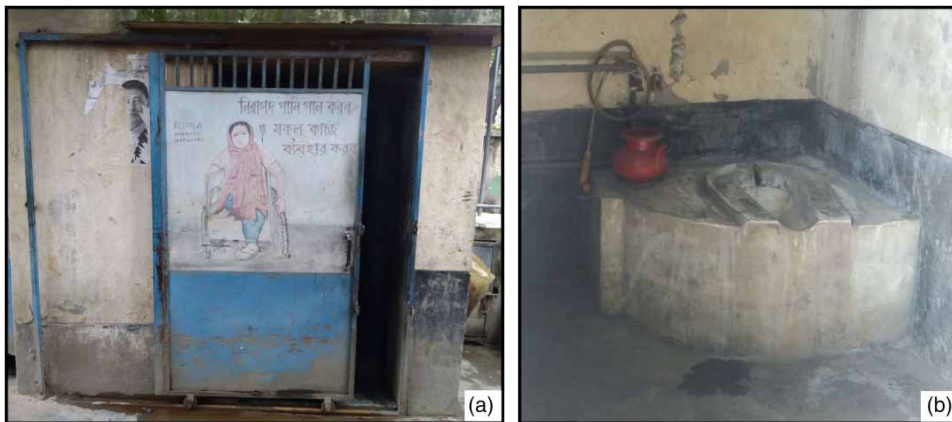
Figure 4 | (a) Disable-friendly toilet but not in working condition due to poor maintenance and (b) common public toilet's pan at high plinth level.
