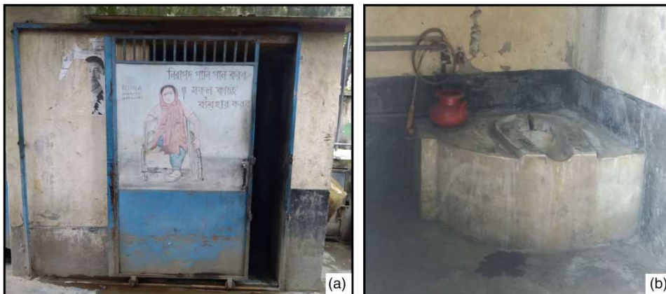
Figure 4 | (a) Disable-friendly toilet but not in working condition due to poor maintenance and (b) common public toilet's pan at high plinth level.
