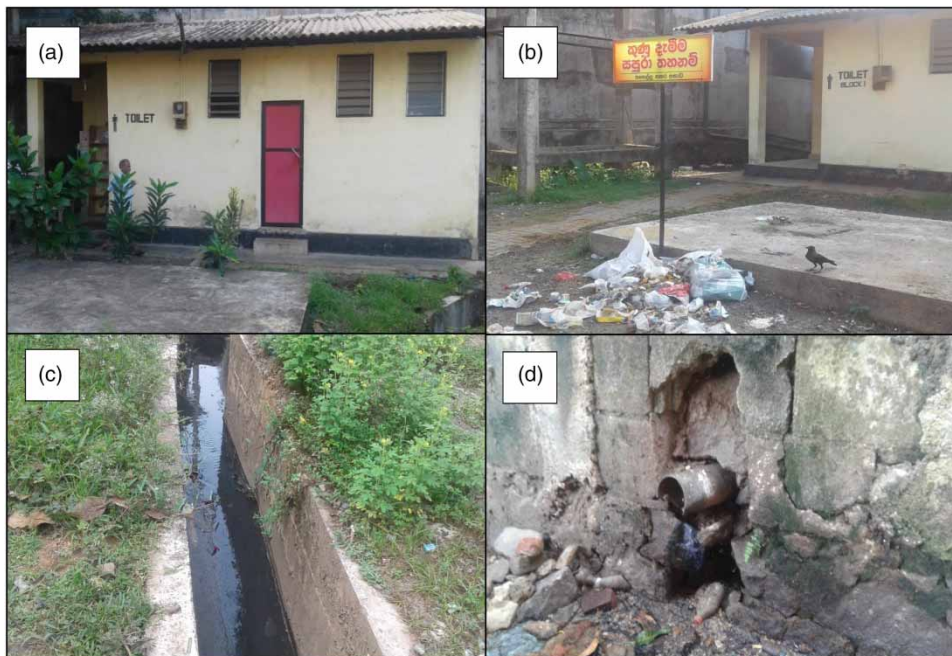
Figure 6 | (a) Existing restrooms at Nidahas Mawatha, Kegalle, (b) improper solid waste management practices associated with public restrooms, (c) poorly maintained drainage near the restrooms, and (d) broken drainage pipelines around the restrooms.
