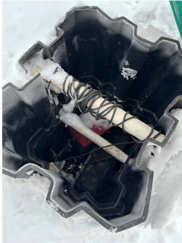
Figure 5 | Opened first compartment of an HDPE septic tank. The photograph was taken at -27 degrees Celsius.
