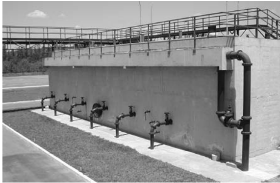
Figure 5.10. View of a full-scale UASB reactor Source: Ipatinga WWTP, COPASA, Brazil
