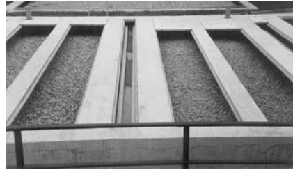
Figure 5.4. Anaerobic filter after UASB reactor (source: Ipatinga WWTP, COPASA, Brazil)
