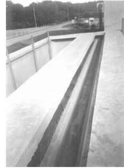
Figure 5.6. Effluent collection launder on the top of an anaerobic filter (Ipatinga WWTP, COPASA, Brazil)
