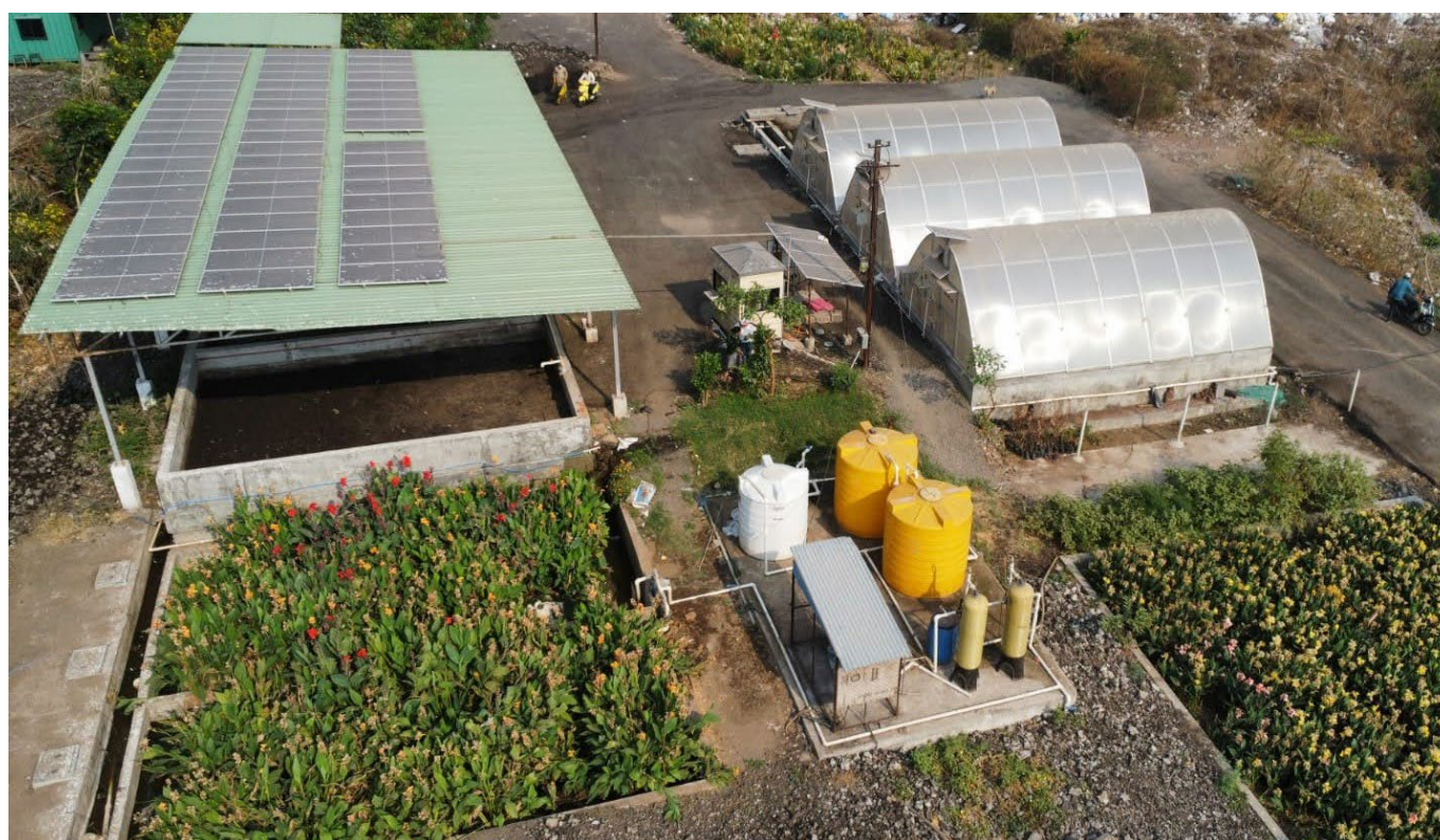
Figure 6: Covered sludge drying bed at Satara faecal sludge treatment plant, Maharashtra 2024 (Image source: CWAS)
