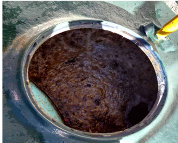
Figure 4 | Formation of a thick scum layer at the settler compartment surface.
