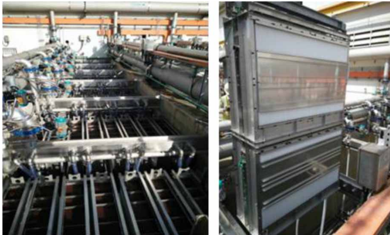
Figure 2 | Pictures of the membrane tank (left) and the membrane unit (right) in CAWW.
