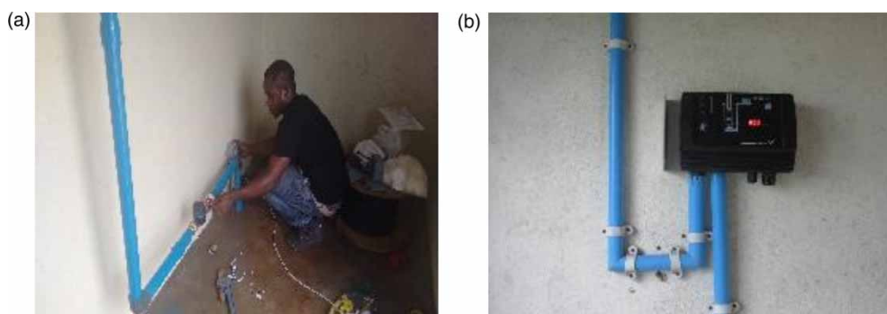
Figure 4 | (a) Satellite water meter and communicator installation (b) CU200 as installed in the enclosure.
