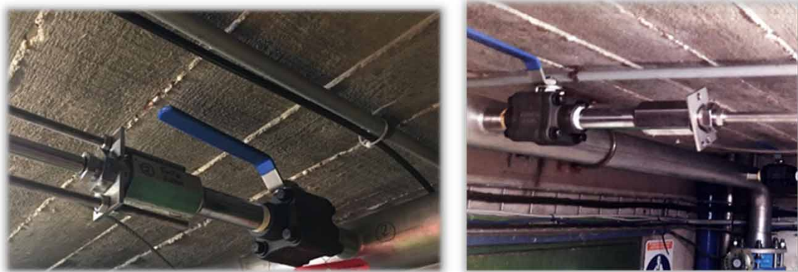
Figure 4 | Online lead and cast iron corrosion probes at plant outlet.
