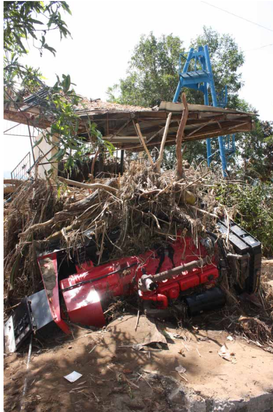
Figure 1 | Damaged genset at Production Well 19, Photograph: COWD.
