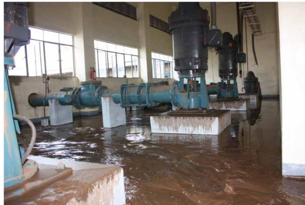
Figure 2 | Flooded booster pumps at Macasandig BPS Photograph: COWD.
