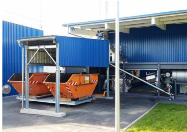
Figure 4 | EloDry-PRO® installation, on the right the PYREG® module, in the building the EloDry-PRO® containers for P-fertiliser ash are visible on the left side.
