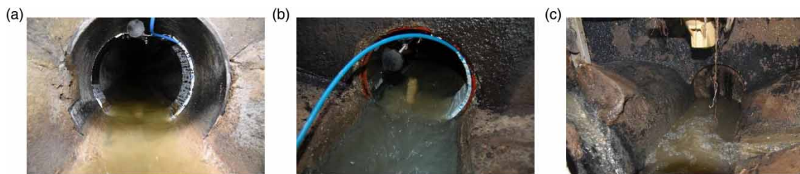
Figure 6 | Examples of sensors poorly installed in sewers. (a) Sensor in a supporting ring, top of the pipe (b) Sensor in a supporting ring, bottom of the pipe (c) Sensor above the pipe, in the manhole wall.
